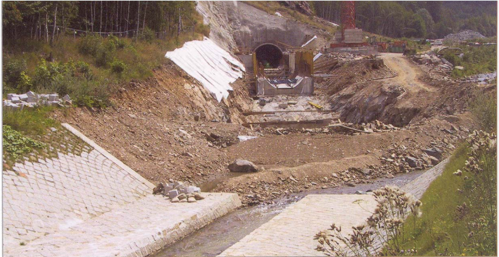
Fig. 13: Construction site for the flood water retention basin above Lauenstein (photo: S. Schümberg 2003)
