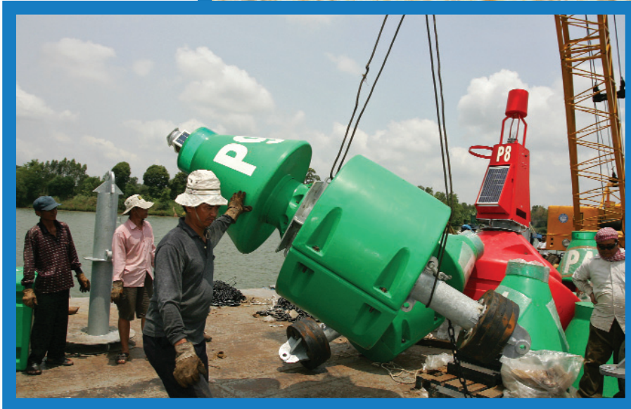
The Navigation Programme has successfully installed a series of buoys, beacons and shoremarks between Phnom Penh Port and the Viet Nam border to assist effective and safe waterborne transport.
