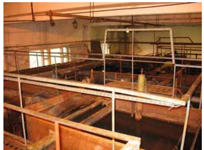
Photo 4. Facilities of the Bondarny WWTF
