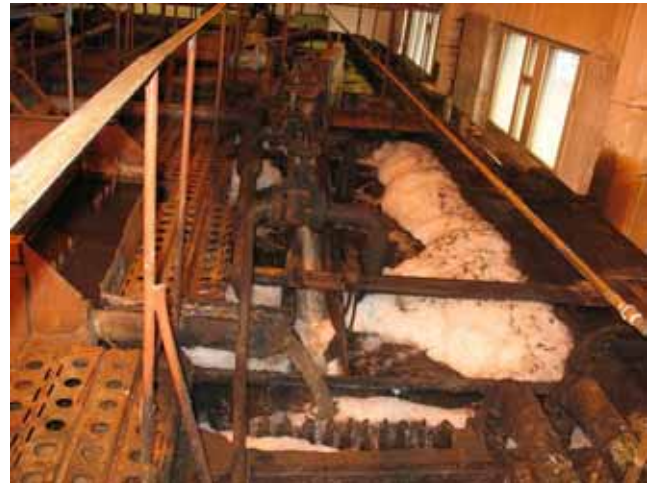
Photo 2. Facilities of the Bondarny WWTF
