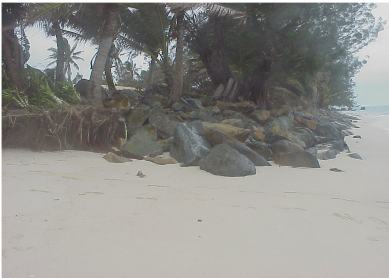
Photograph 12.0 An example of a improperly built rock revetment.
