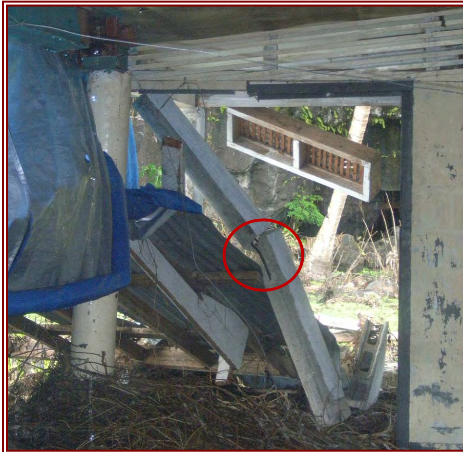
Figure 40: Two lengths of vertical rebar were exposed in a broken column showing its poor spacing and insufficient lateral reinforcement
