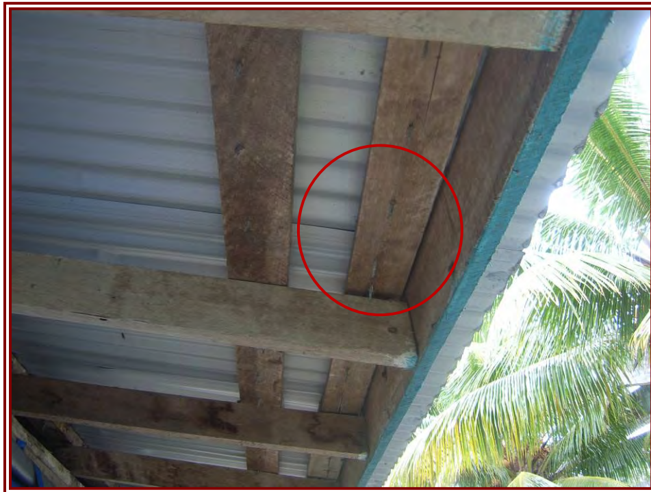
Figure 41: Nails protruding through a corrugated iron roof to underlying timber beams
