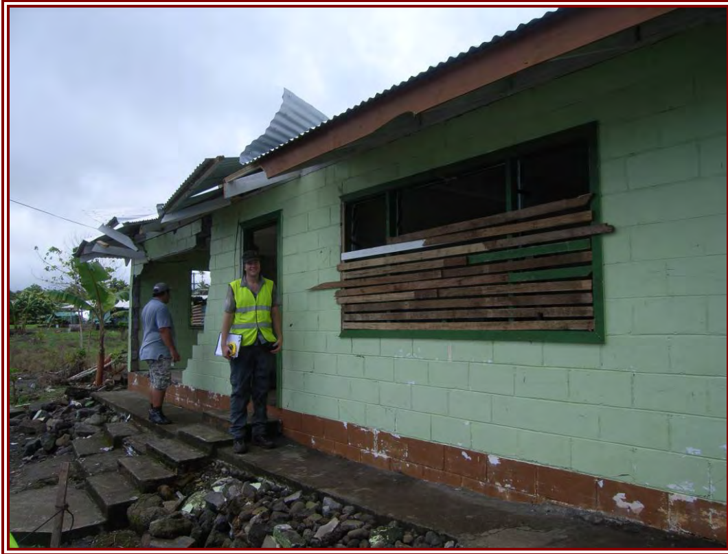
Figure 16: This reinforced concrete frame house built in 2007 had damage to the front and back infill walls. All partition walls inside was also damaged, although the structure remained standing.
