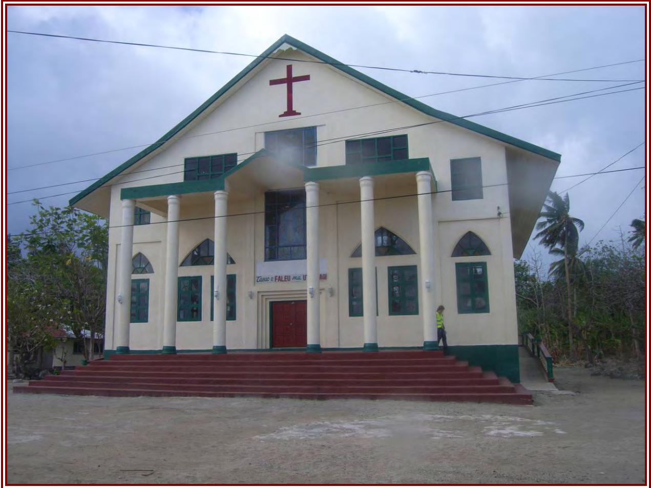
Figure 33: No damage was evident at this reinforced concrete frame church at Lepuia'i. As observed in many of the surveyed villages, churches, possibly better built fared much better than other structures.
