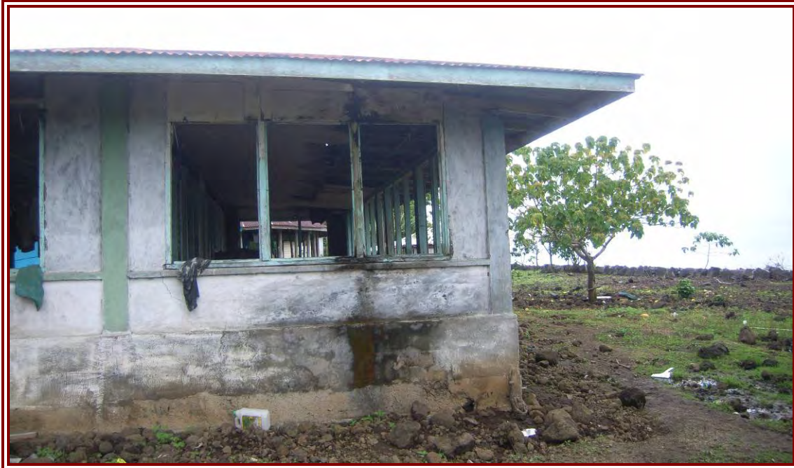
Figure 37: The incoming water had lifted the floor of the concrete foundation to this residential building, although the foundation was 80cm high
