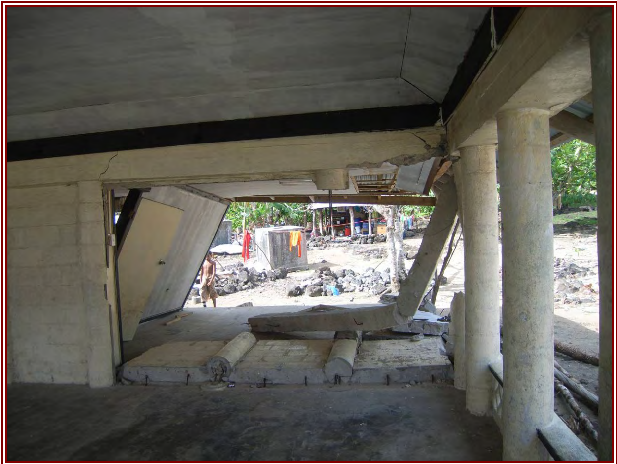
Figure 32: Damage to the weakly reinforced concrete columns and infill walls of a house at Lepuia'i
