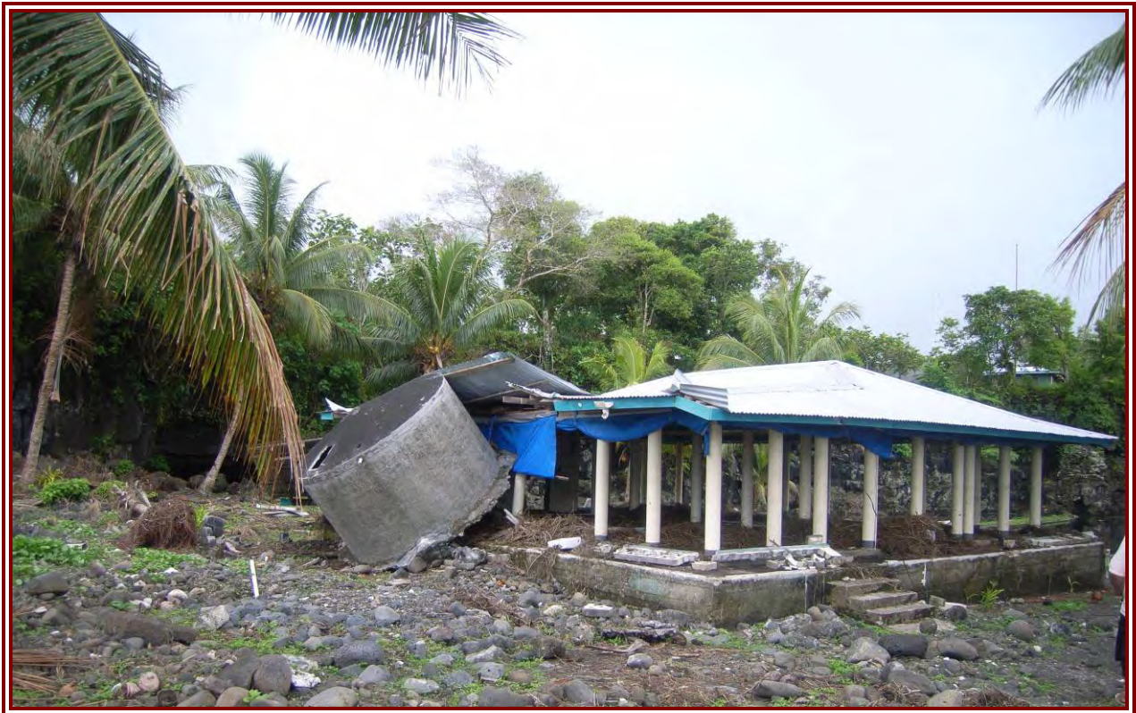
Figure 39: A photograph showing the impact of a displaced concrete water tank on an open reinforced concrete column building at Taga
