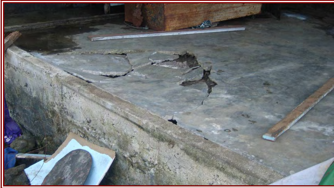
Figure 35: Evidence of lifting of concrete floors as water rose through foundation and ruptured concrete blinding (usually <20mm thick)
