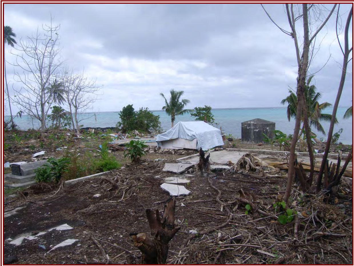
Figure 30: The remains of a timber fale at the village of Lepuia'i completely destroyed by the tsunami wave; only the concrete base foundation remains.
