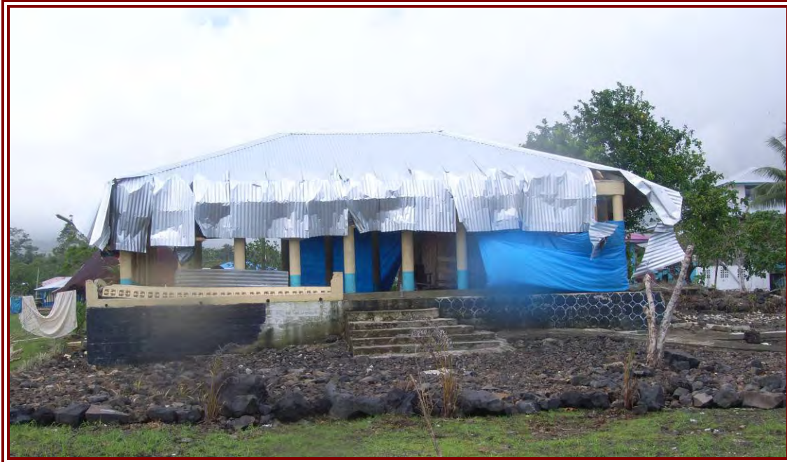
Figure 17: This photograph would suggest the wave may have impacted from above as the corrugated iron roof was bent downwards
