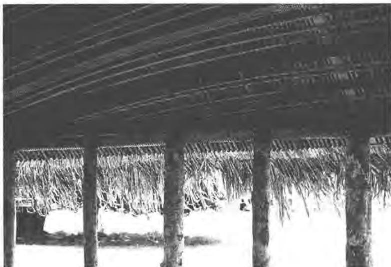
The new 'fale' at Samoa College, Apia, replaces the previous 'fale' destroyed by Cyclone Val. Built in traditional style, synthetic twine replaces the coconut sennet. (photo: A.C. Robinson, reproduced courtesy of DLSE)
