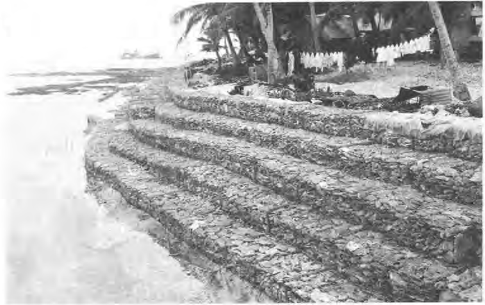
Sea wall on Nukunonu built to prevent further erosion caused by cyclones.
