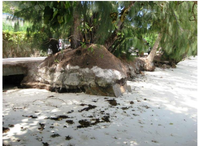
Figure 12: Beach erosion is becoming a more common problem
