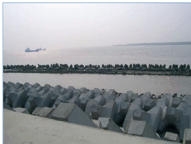
Dikes along the Yangtze coast designed to prevent coastal erosion from reduced sediment input, typhoons and high tides (Photo: M.T. Li)
