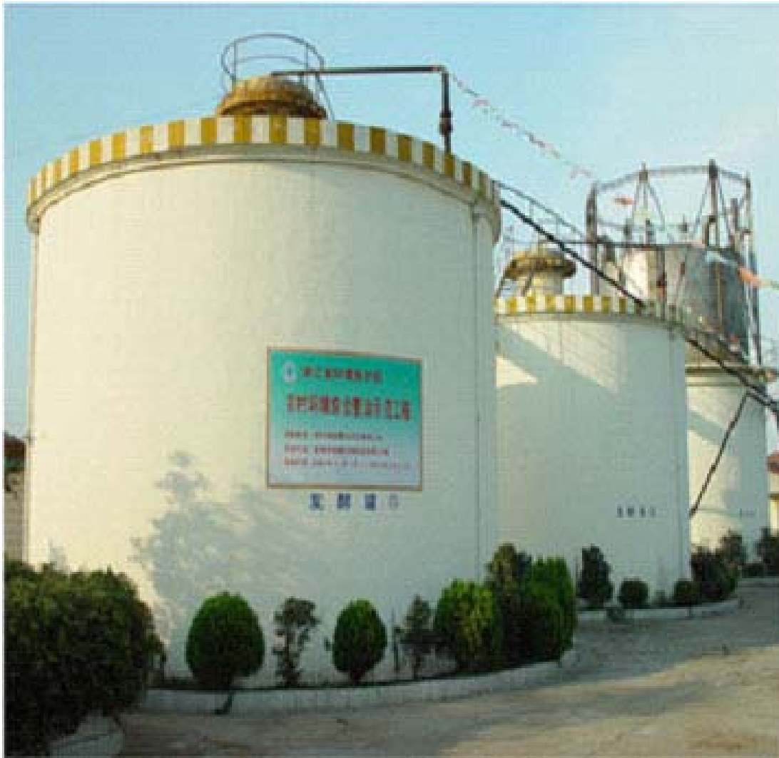
Modified UASB tanks
