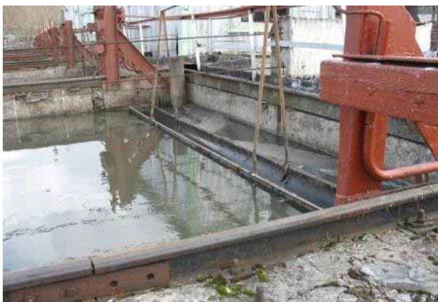
Photo. 7. Primary horizontal sedimentation tanks with a gear to collect floating contamination
