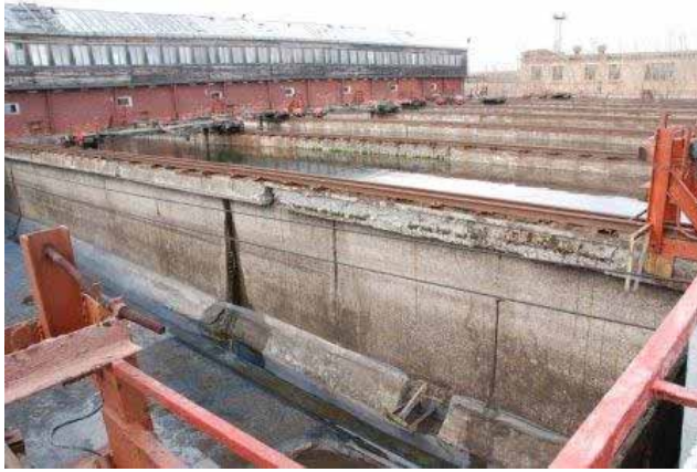
Photo. 1. Secondary horizontal sedimentation tanks
