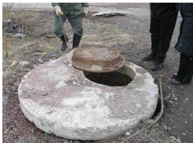
Photo 4. Well with faulty floor slab and untight manhole
