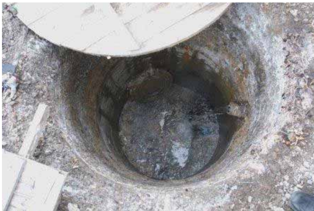
Photo 1. Well without floor slab, cover at the bottom
