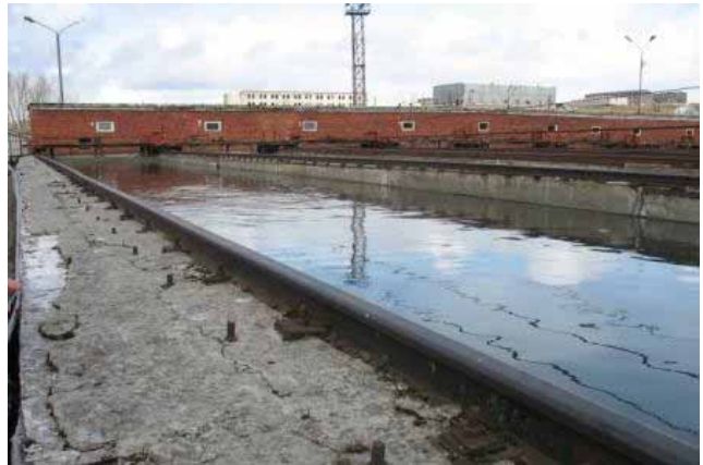
Photo. 4. Primary horizontal sedimentation tanks
