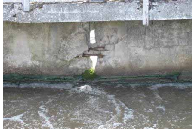
Photo. 2. Faults of reinforced concrete walls of active sludge tanks
