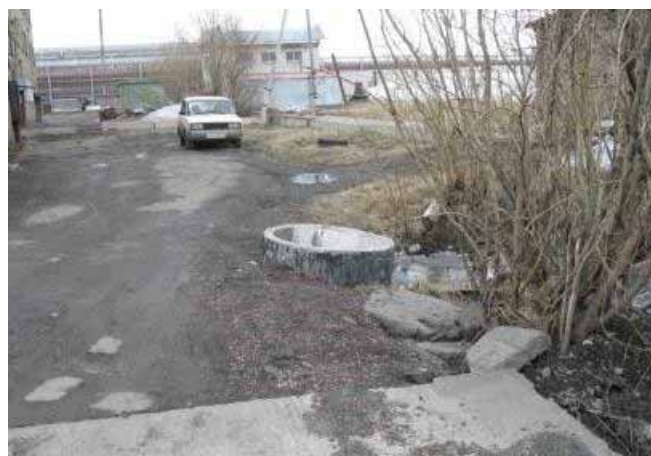
Photo 6. Well without floor slab and filled with water
