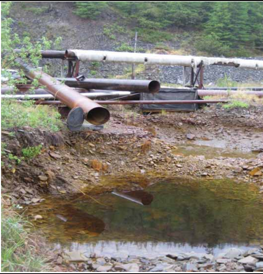
Photo 5 Outlet for discharge of water via the siphon system to the Poiskovy Stream. Water is discharged without required permits.
