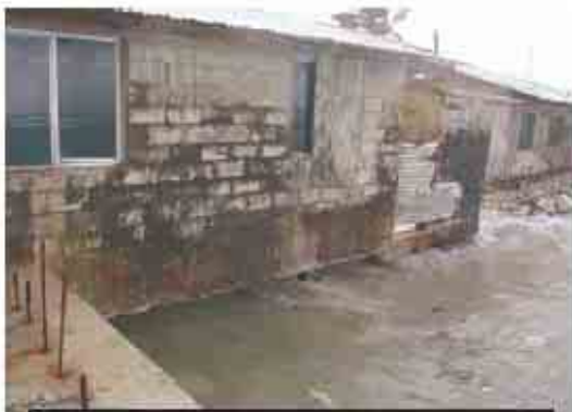
Incoming waves under house (bathroom already collansed)
