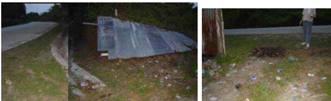
NE view showing fallen corrugated fence and swale for road.
