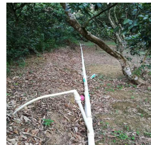
Biogas slurry utilization pipe network
