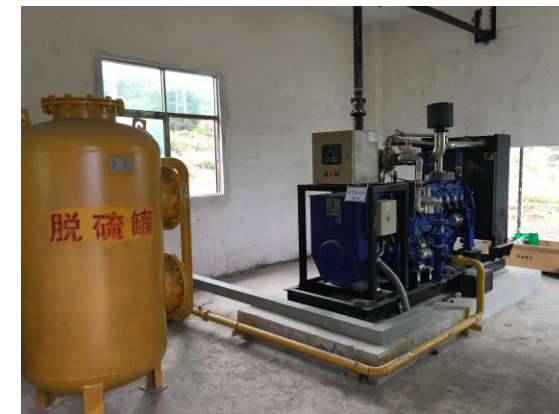
Biogas power generation set
