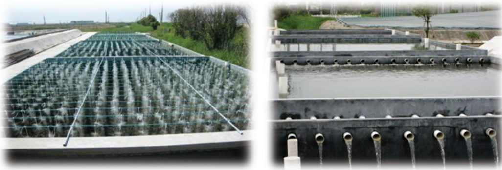
Figure 3-16 The quadropole tandem farming discharged water sedimentation tank in the discharged water treatment system. (Zhejiang Mariculture Research Institute)
