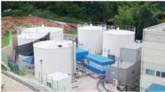
Land-based facilities for testing ballast water treatment devices
